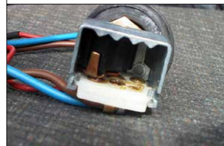
Broken Light Switch
